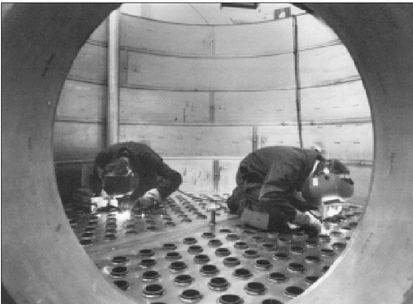
Heat exchanger inlet section thin-sheet lined with HASTELLOY C-276 alloy.
