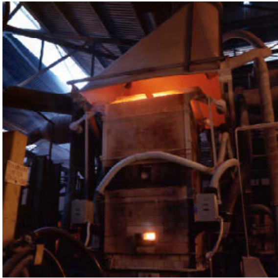
HAYNES® 230® damper atop this glass melting furnace withstands 2300°F (1260°C) for short times and 2000°F (1093°C) for sustained periods.
