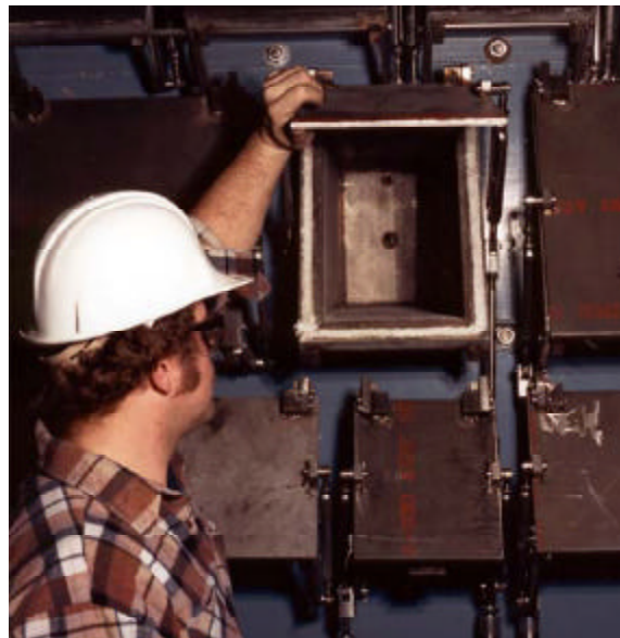
230 retorts operate at 2100°F (1149°C) with a hydrogen atmosphere (inside) and combustion products outside.
